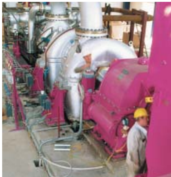
31MW Allen Steam Turbine installed at Møljervaerket Combined Heat and Power Plant in Denmark during overhaul.
